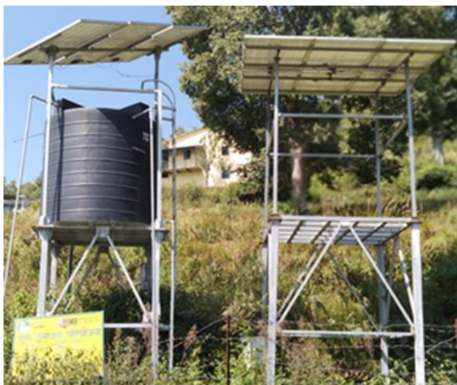
Solar based pumping Scheme
